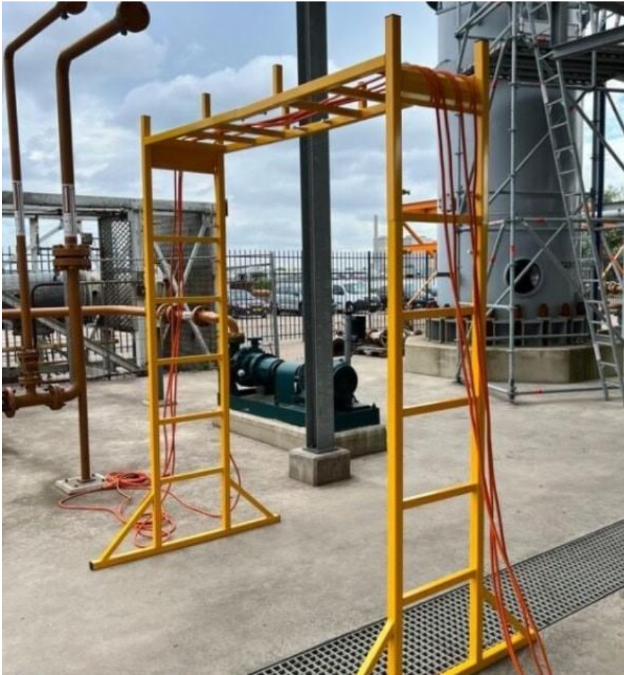
Cable Bridge to suspend cables over a walkway
